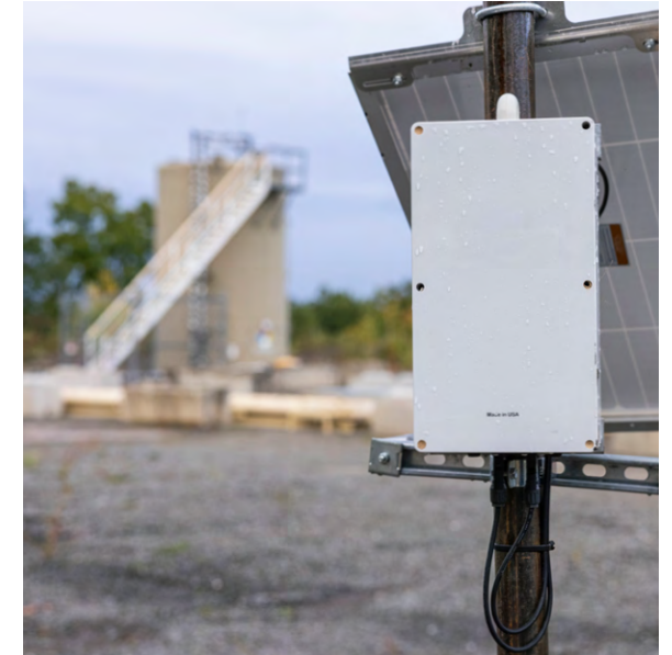
In our Haynesville and Marcellus operating areas, we utilize fixed methane monitoring technology to detect emissions at our production sites. More than 2,000 sensors are deployed across our assets.
